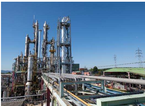
Speichim Processing (France)
