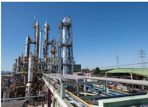
Speichim Processing (France)
