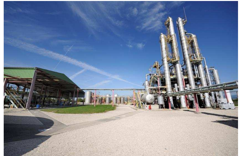
Chemical purification – Speichim Processing
